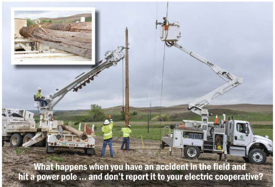
From left: Journeyman Lineman Blake Reis (operating digger-derrick), Leadman Clint Begger (holding plumb bob), Journeyman Lineman Brady Zachmann (tamping dirt) and Leadman Jason Jahner (waiting to reattach power line, from bucket) worked the line hot to avoid disrupting power to the member.
