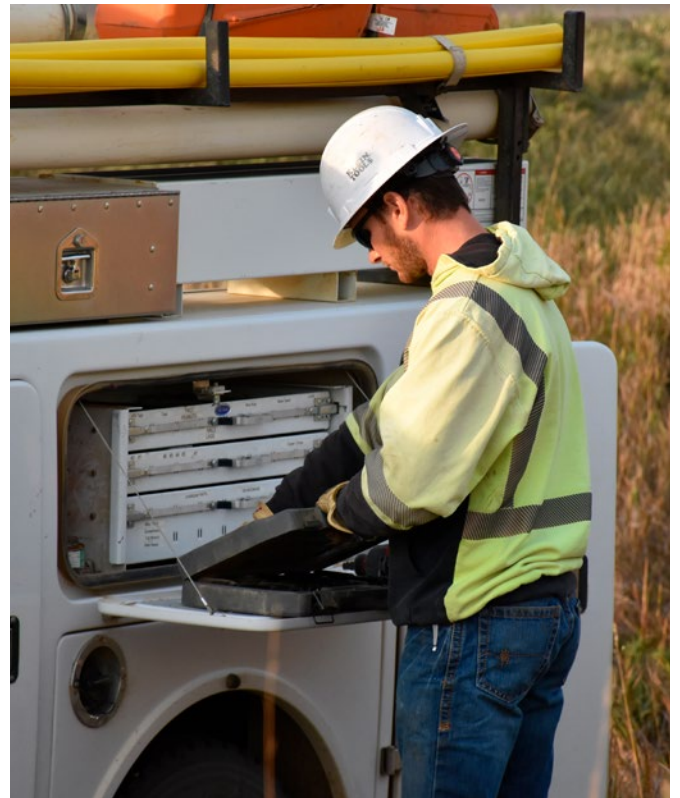
Wayde Eckroth , journeyman lineworker grabs tools from the line truck while working on a project in northwest Mandan.
